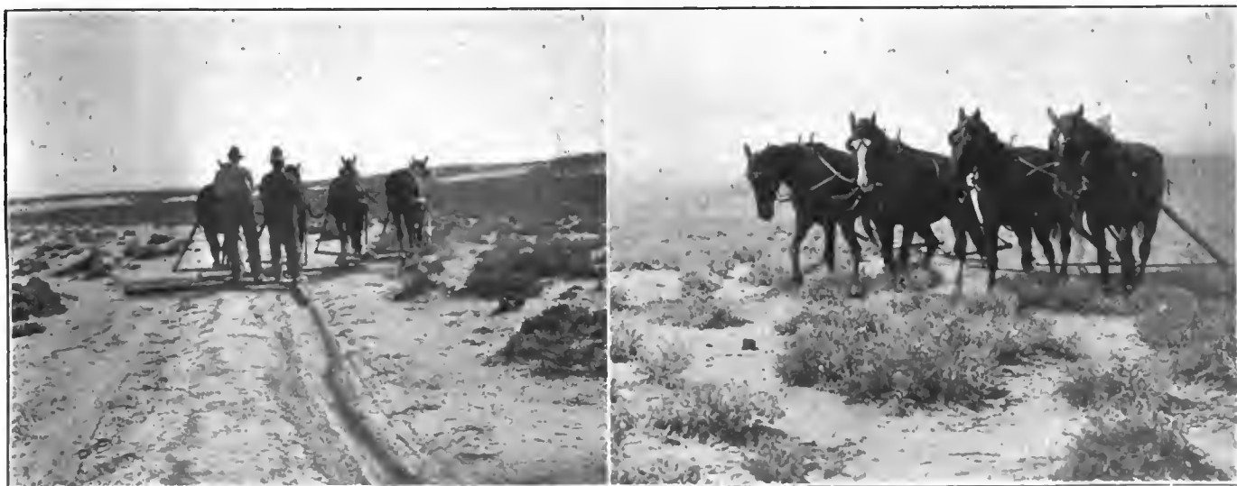
Left—Starting the work on the new roadway south of the railroad grade in Northwestern Utah. A steel rail, used either in its normal straight line or else bent into V-shape, is pulled by four horses to tear out the sage brush and other growth. For the first attack a straight rail gives a greater strain. Right—After sage brush has been railed out by its roots to the desired road width, then comes the shaping of the road by crowning for drainage.
